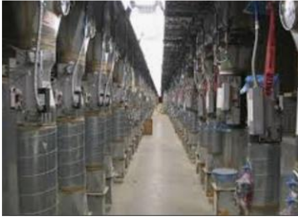
Figure 26 State-of-the-Art White Oak Infrastructure: Advanced Air Terminal Units Supporting Laboratories
